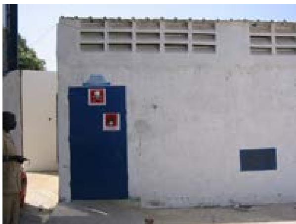
Example of a well-protected and well ventilated storeroom. Note the safety pictograms on the door. (Photo B. Schiffers)
