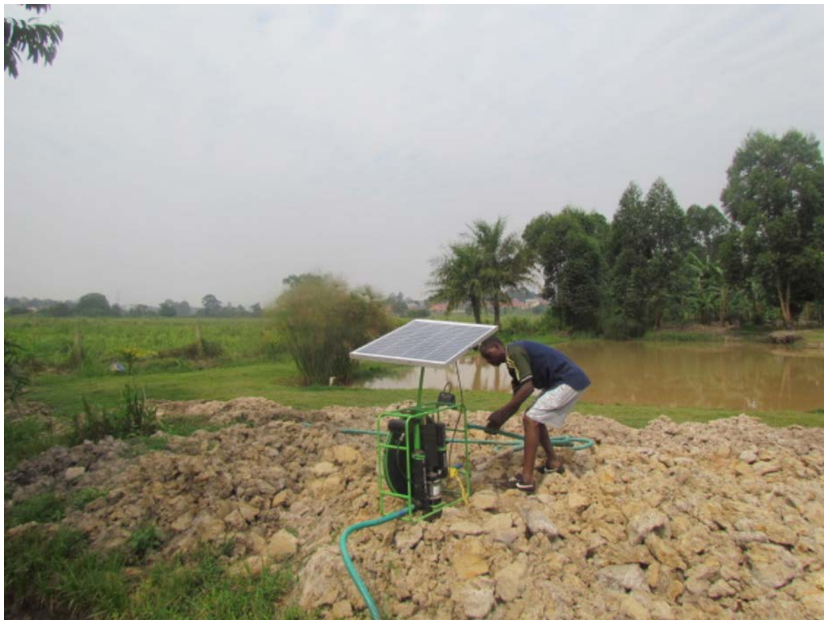
Figure 7 - Simple solar powered water pump - no source
